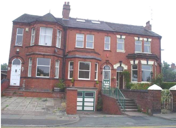
FIGURE 22: Harmful modifications where front walls and gardens have been removed on two properties. One has also had its chimney stack removed and had roof lights inserted, while two have lost their original windows.
