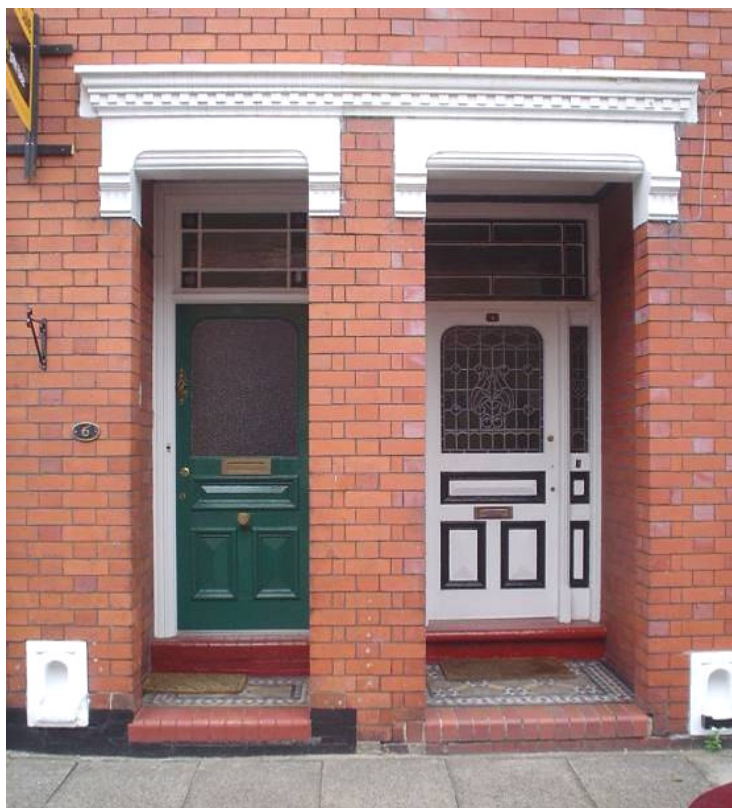
FIGURE 14: Porches, doors and boot scrapers. Nos. 4 and 6 Wilfred Place preserve a range of original features. The stained glass insets of No.4 provide a point of interest.
